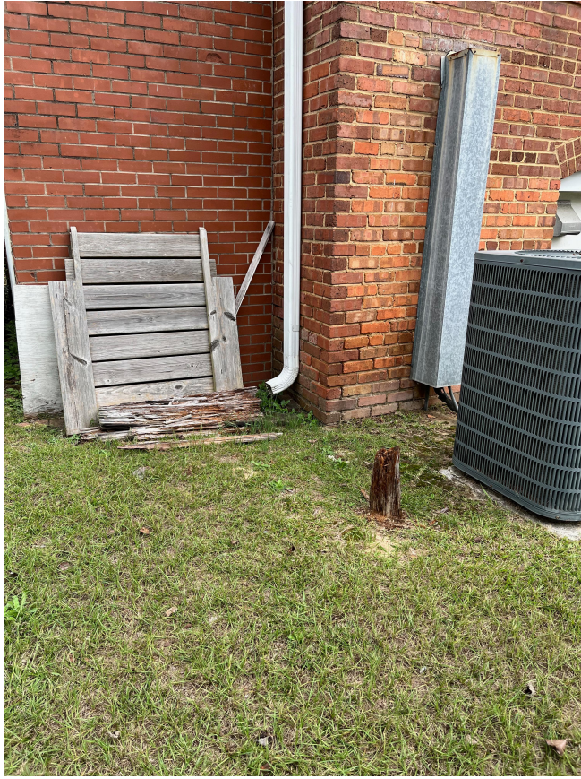
Existing Condition: Downspout without rain leader
