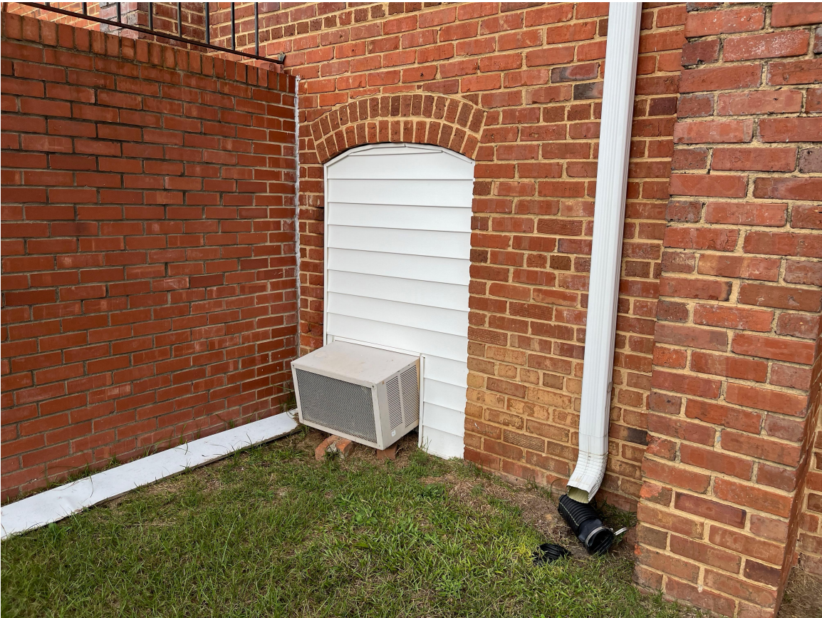
Existing Condition: Downspout without rain leader
