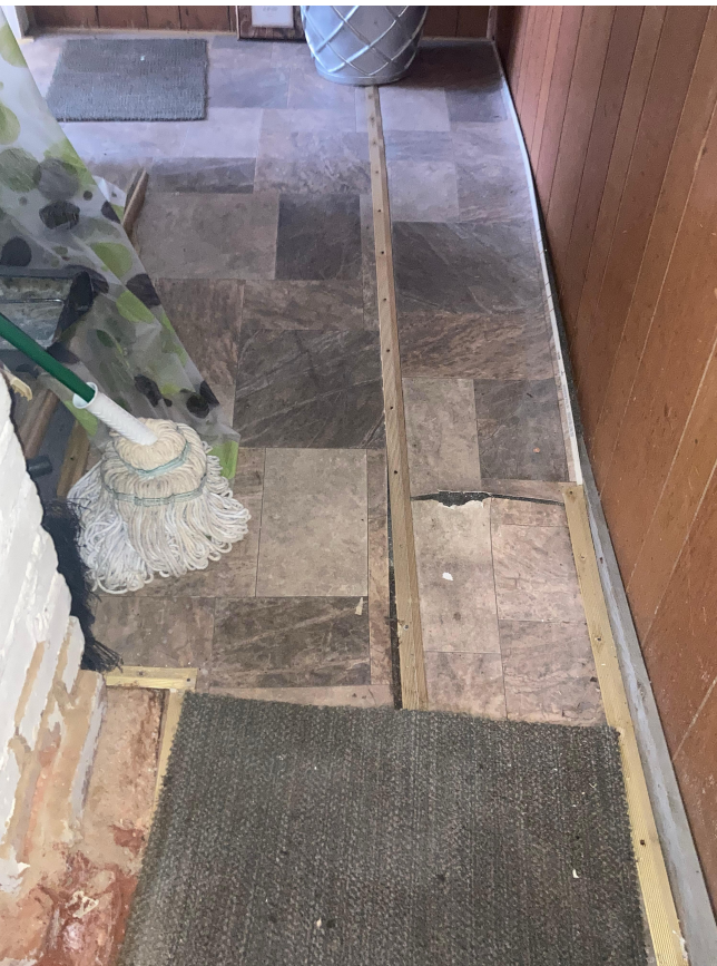
Existing Condition: Uneven flooring in basement hall
