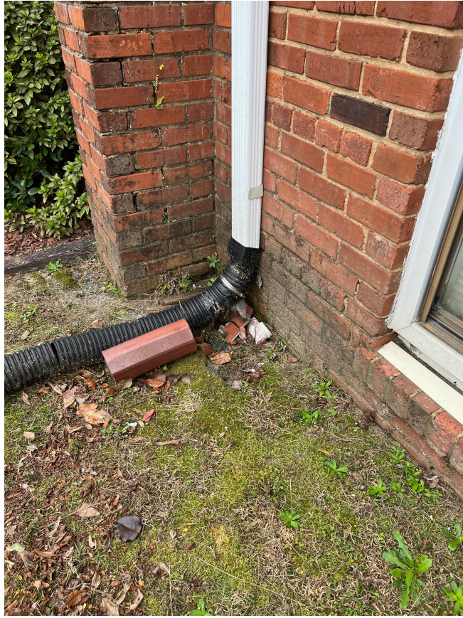
Existing Condition: Downspout damaged rain leader
