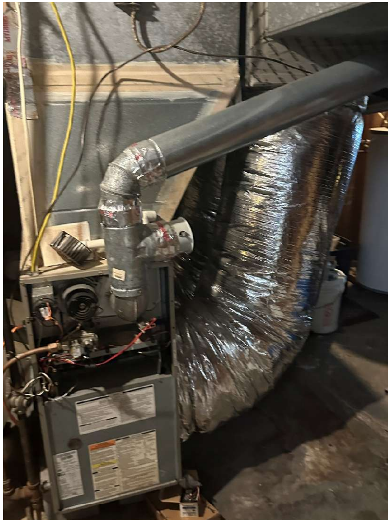
Existing Gas Furnace
