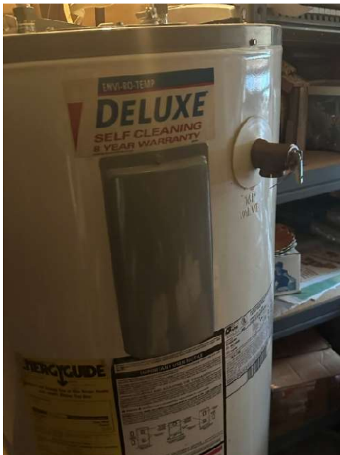
Existing Water Heater
