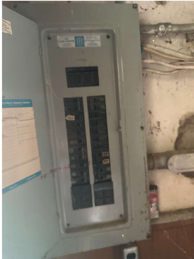
Existing Electrical Panel
